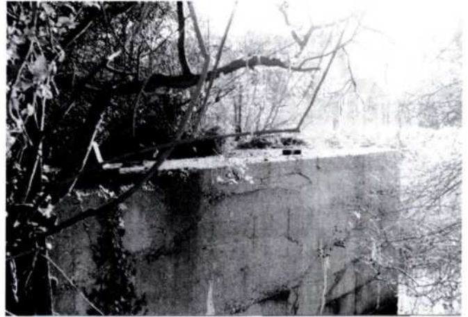
Fig. 5 The west face of the Chichester abutment in 1984 showing the burnt-off remains of the portal frame and part of a winch. (Author)
