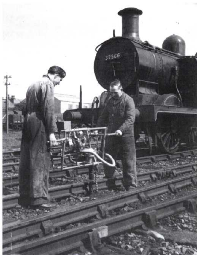
Fig. 7 A petrol-driven drill built for British Rail by H.A. Waller & Sons. A petrol-driven saw to cut through the rail-track was, among others, a companion device. (S.W. Kenyon)
