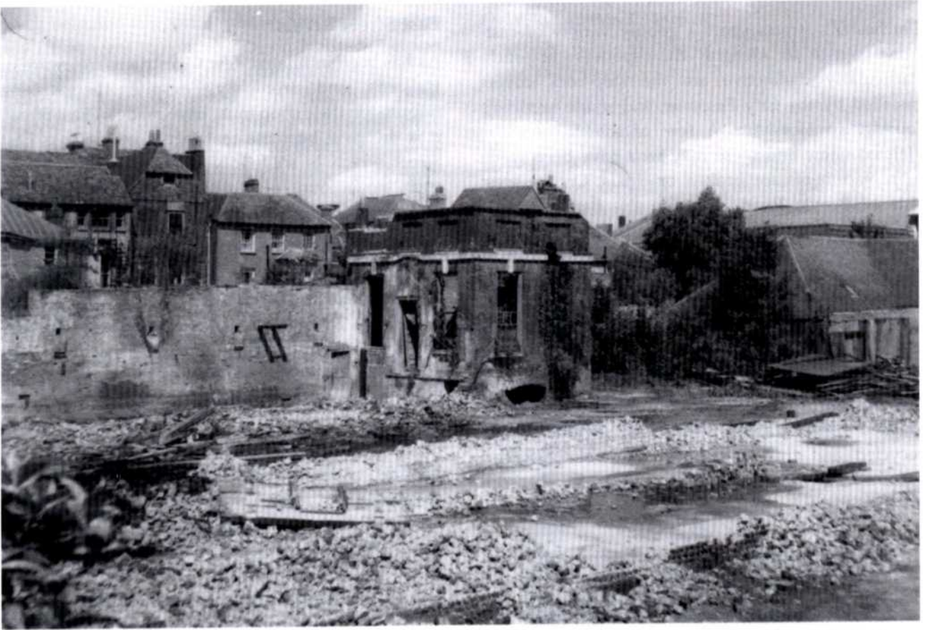
Fig. 16 Demolition of the north range of buildings in 1960. Only the north wall and the furnace house are still standing. In the foreground the piles of flints mark the site of the middle range. (WSRO)
