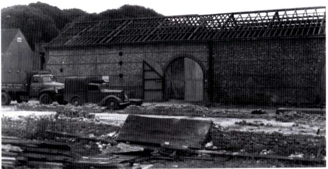
Fig. 17 Demolition of the south range in 1960. The flint and brick buildings were quite substantial – and not unattractive. To the left of the building can be seen the entrance from East Pallant: the building over the top of it had already gone.(WSRO)
